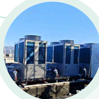
▲ Application of air source heat pump technology
