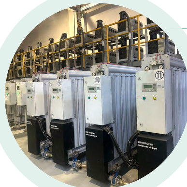
▲ Adsorption-type vacuum-assisted heating dryer
